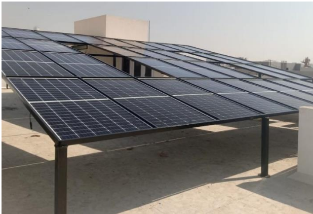
Pipe Based Elevated Structure
